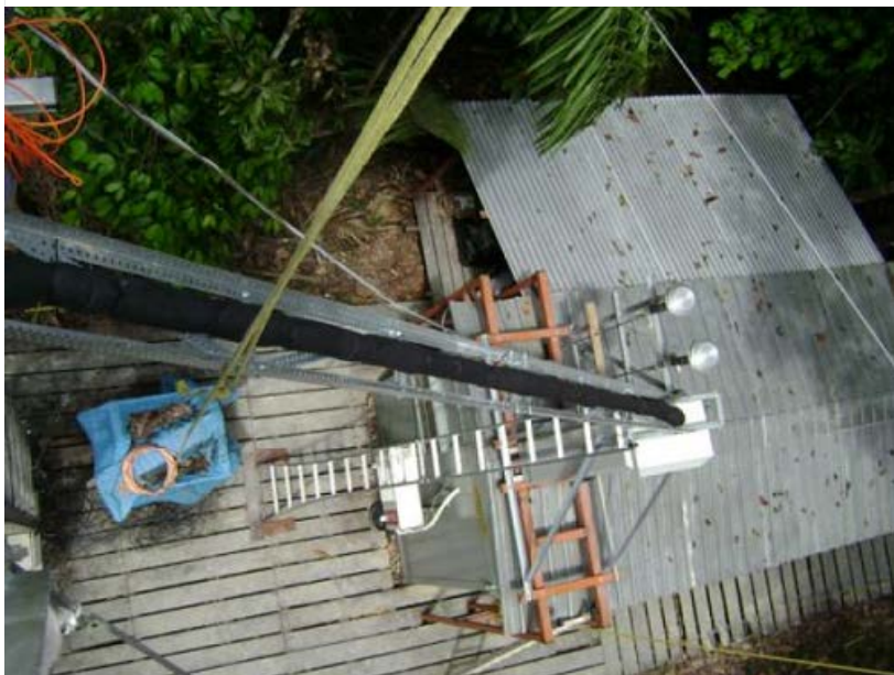
Figure 3. Close-up view of the lower part of tower looking at horizontal connector of sampling line.
