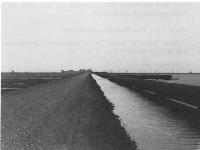
Figure 82. Ponding caused by damming effect of the road.
